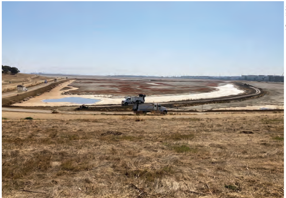
Thanks to the generosity of Pacific States Environmental, in partnership with California Wildlife Foundation, millions of cubic yards of clean, tested soil have been delivered to this and other South Bay restoration sites, saving state and federal partners millions of dollars.
